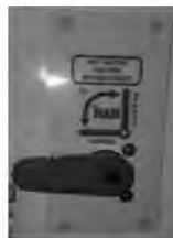
Water Heater Bypass
