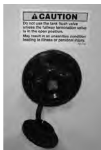
Tank Flush Inlet
