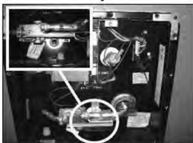
Fig 1: Water Heater Drain Plug
