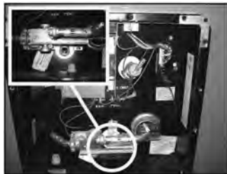
Water heater drain plug
